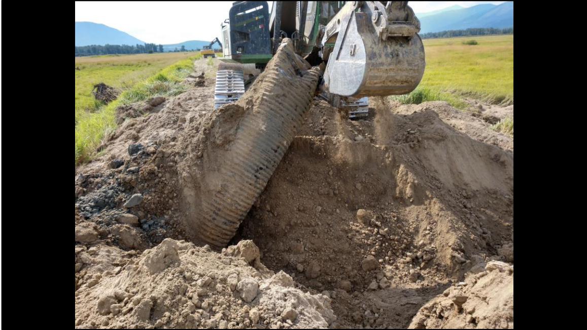
Pipes installed for the impoundment were removed as part of the restoration project. Here a drainpipe and water control structure are being removed.
