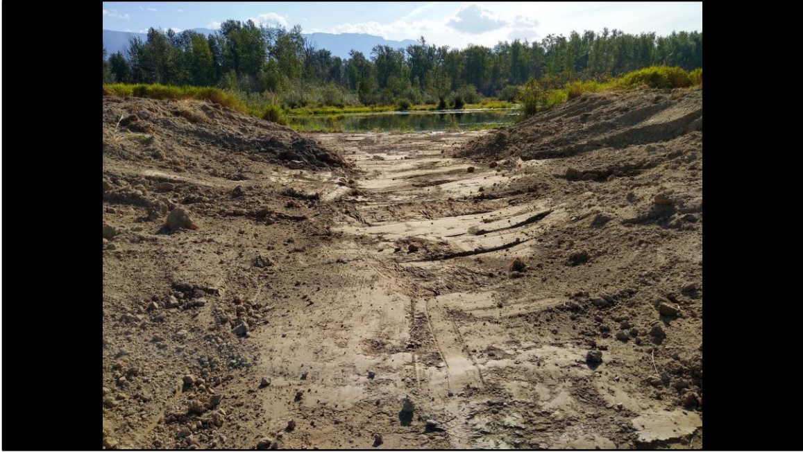
The banks of the restored inlet are sloped after the channel is dug.
