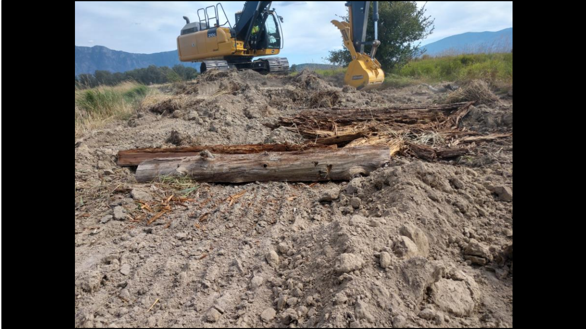
Woody debris uncovered during the removal of the dam was saved and placed by the excavator.
