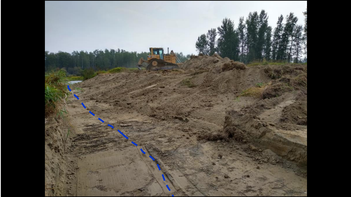
A dozer was used to spread the soil removed from building the inlet. The center of the inlet being restored is shown by the dashed blue line.
