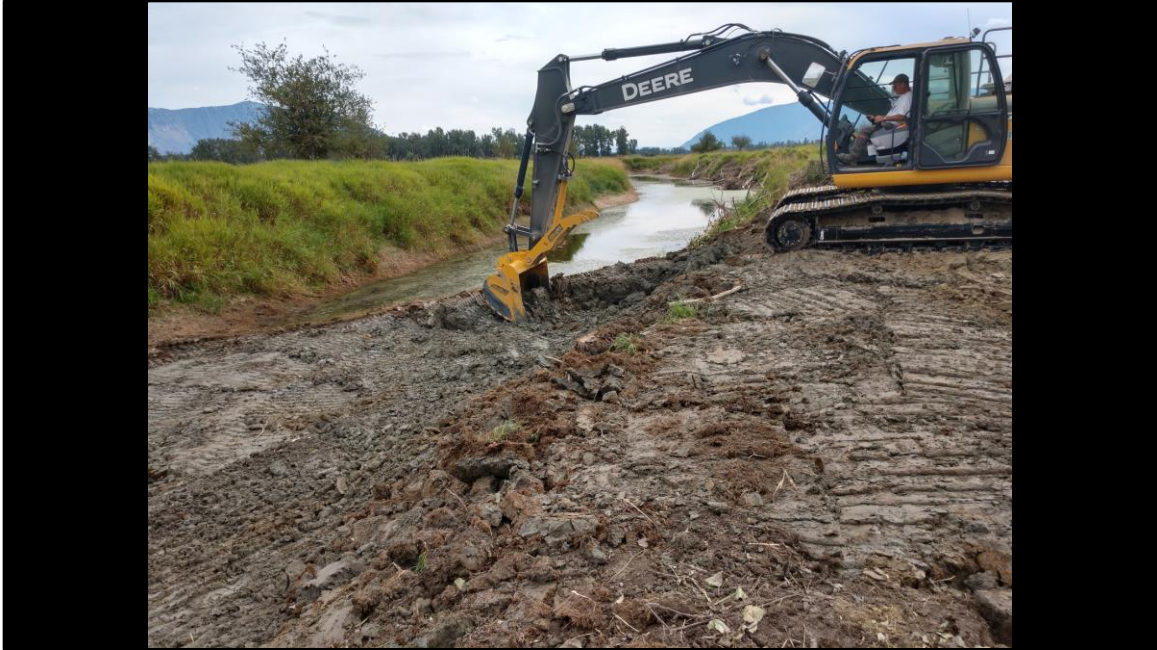
Here the soil that was used to block the natural channel of the Goat River South is being removed by using a John Deere 210G Excavator.
