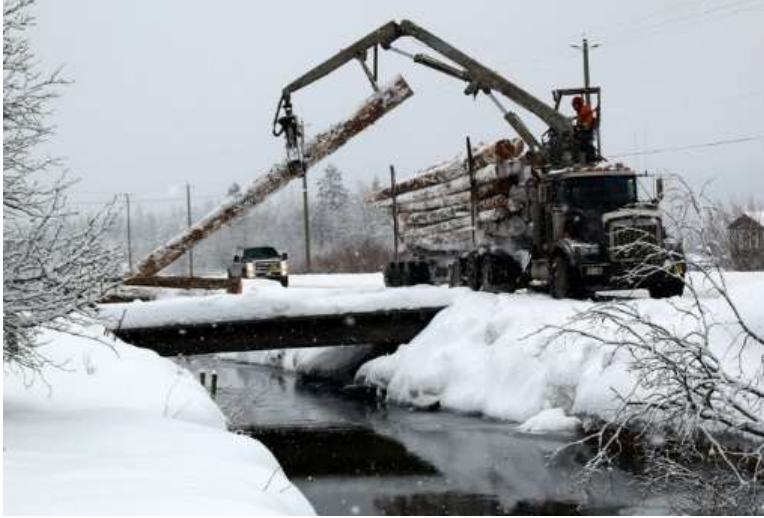
Here a logger uses a self-loader to unload 45-logs at a wetland restoration site.
